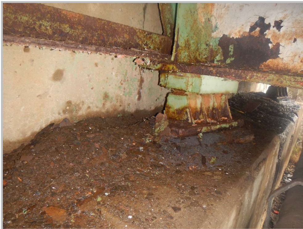
LEAKAGE UNDER FORWARD ABUTMENT JOINT
