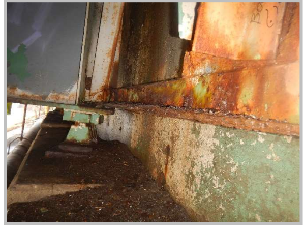
ABUTMENT END CROSSFRAME WITH SECTION LOSS
