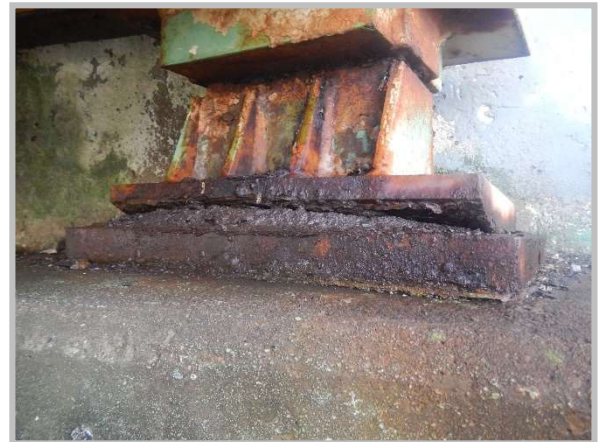
ABUTMENT ROCKER BEARING WITH PACK RUST
