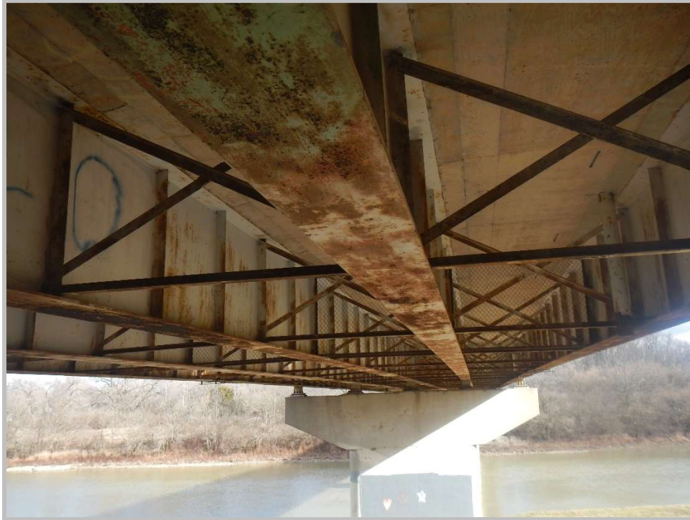
BRIDGE DECK UNDERSIDE, STEEL GIRDER BOTTOM FLANGE RUSTED
