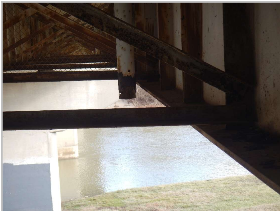
RUSTED SCUPPER DOWNSPOUT PIPE END
