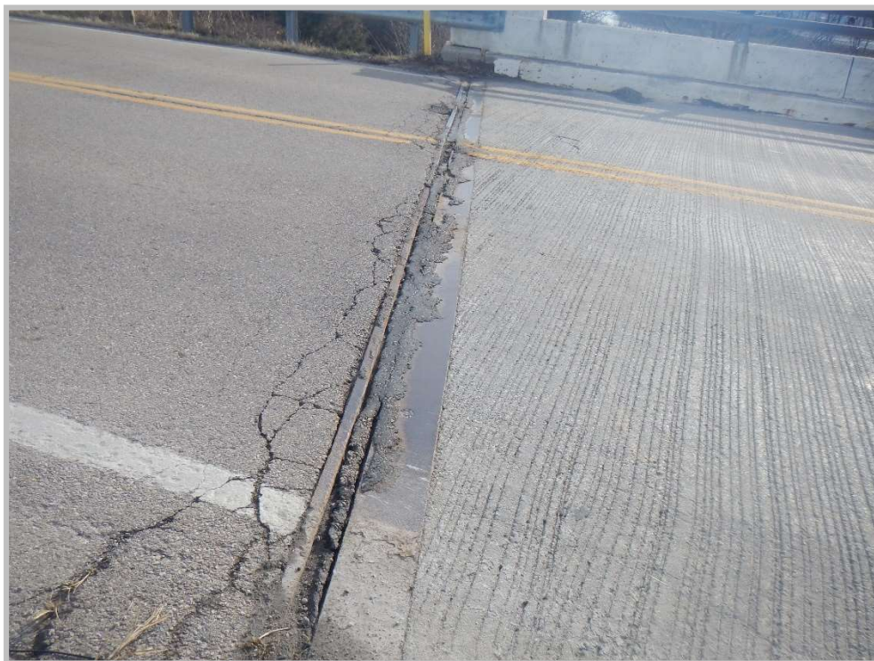
DETERIORATED ABUTMENT JOINT
