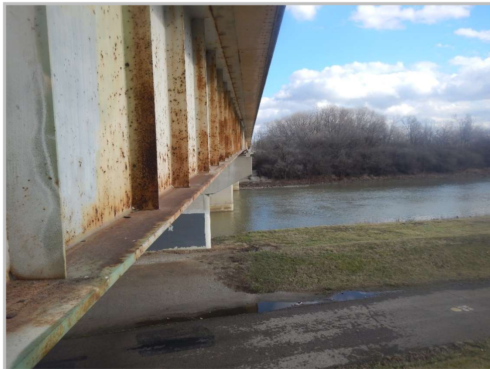
EXTERIOR GIRDER WITH PAINT FAILURE AND ASSOCIATIVE RUST
