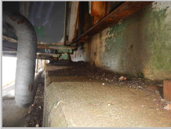
ABUTMENT SEAT AND BACKWALL WITH EVIDENCE OF JOINT LEAKAGE
